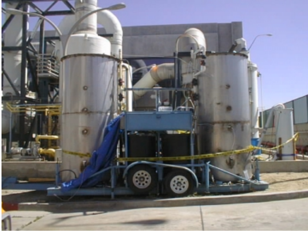
Figure 5. Picture of the UCR biotrickling filter installed at Hyperion Wastewater Treatment Plant in Los Angeles..
