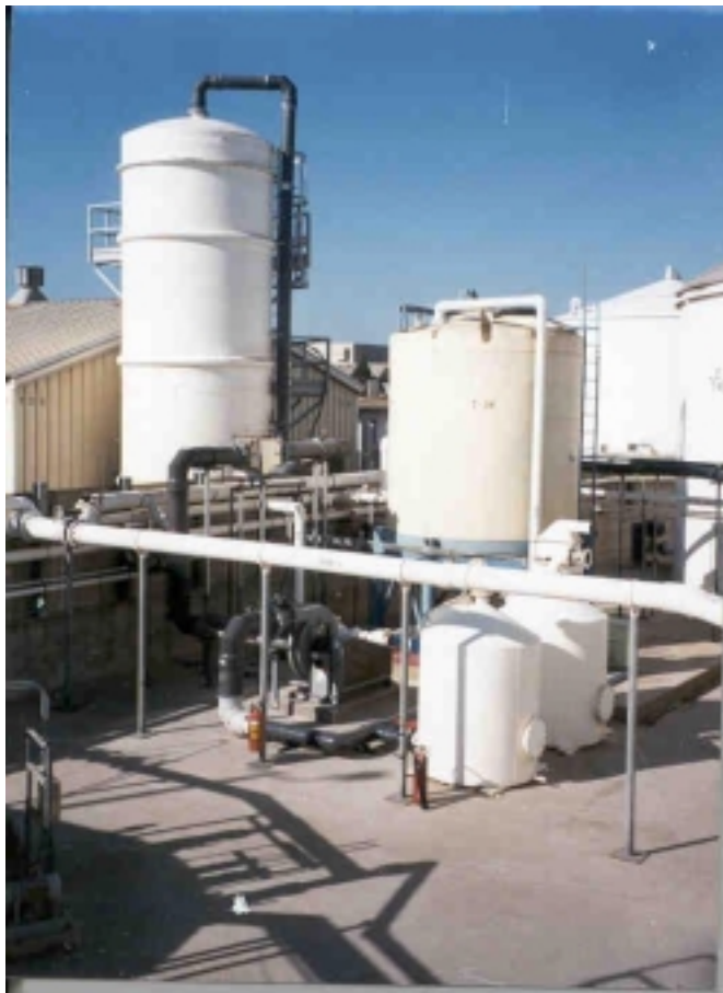
Figure 8. The North Island - Naval Air Station biotrickling filter (Courtesy of Todd Webster, Envirogen Inc.).
