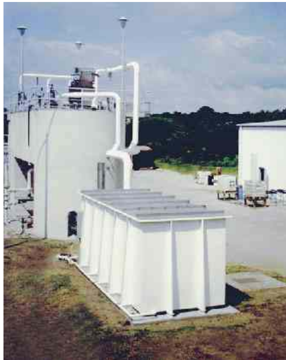
Figure 6. Picture of an actual biofilter. The in-vessel system treats H_2S and other odours at a wastewater treatment facility. The EBRT is 20 s. (Courtesy of Biorem Technologies, Inc.)
