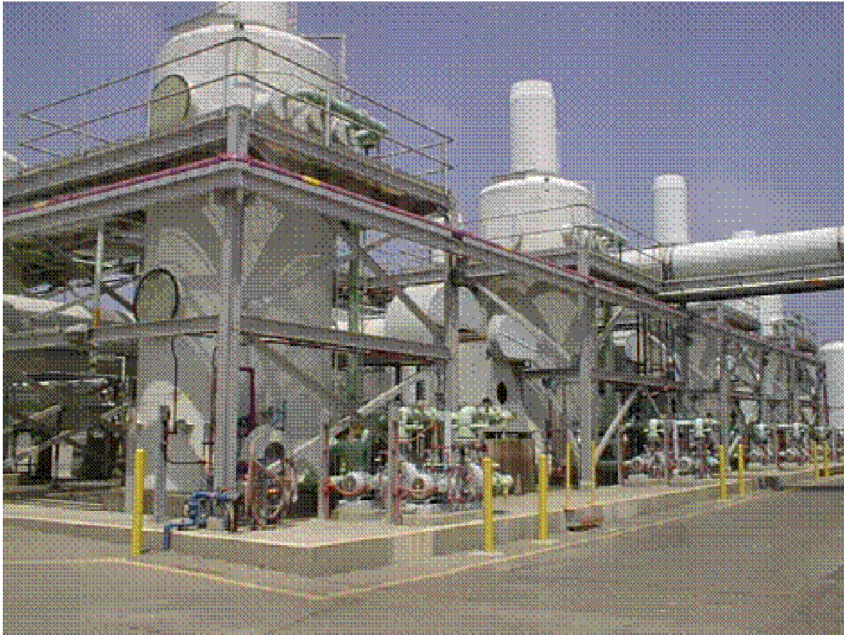
Figure 1. Photo of a bank of eight wet scrubbers at Plant 2 of OCSD. The second from the left has been converted to biotrickling filter Q.
